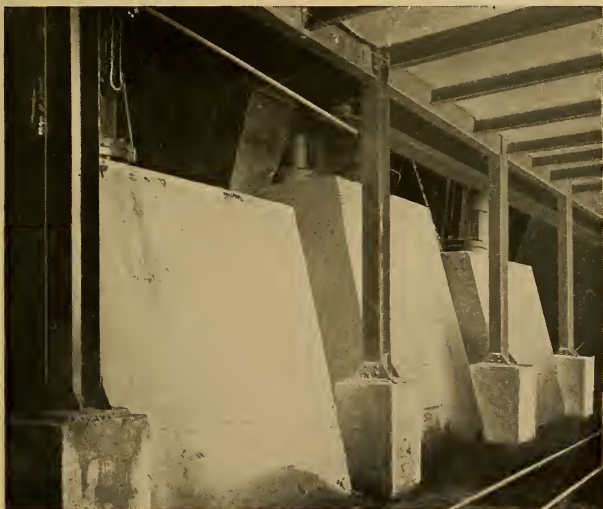
Fig. 157. View showing Several Jolt-Ramming Moulding Machine Foundations with Piers built on the Basement Floor.
